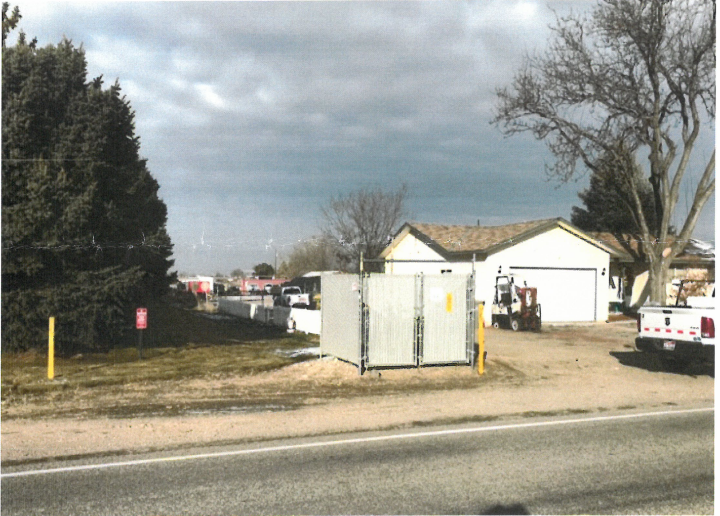
Figure 6: Line Markers at Regulator Station 40107
