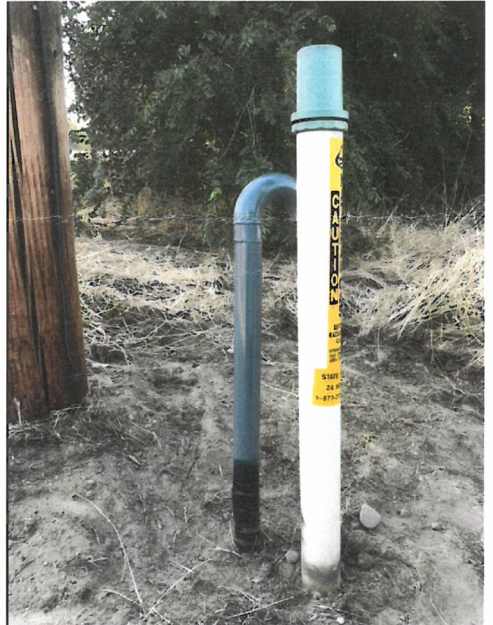
Figure 5: Vent Stack for Casing 26701309
