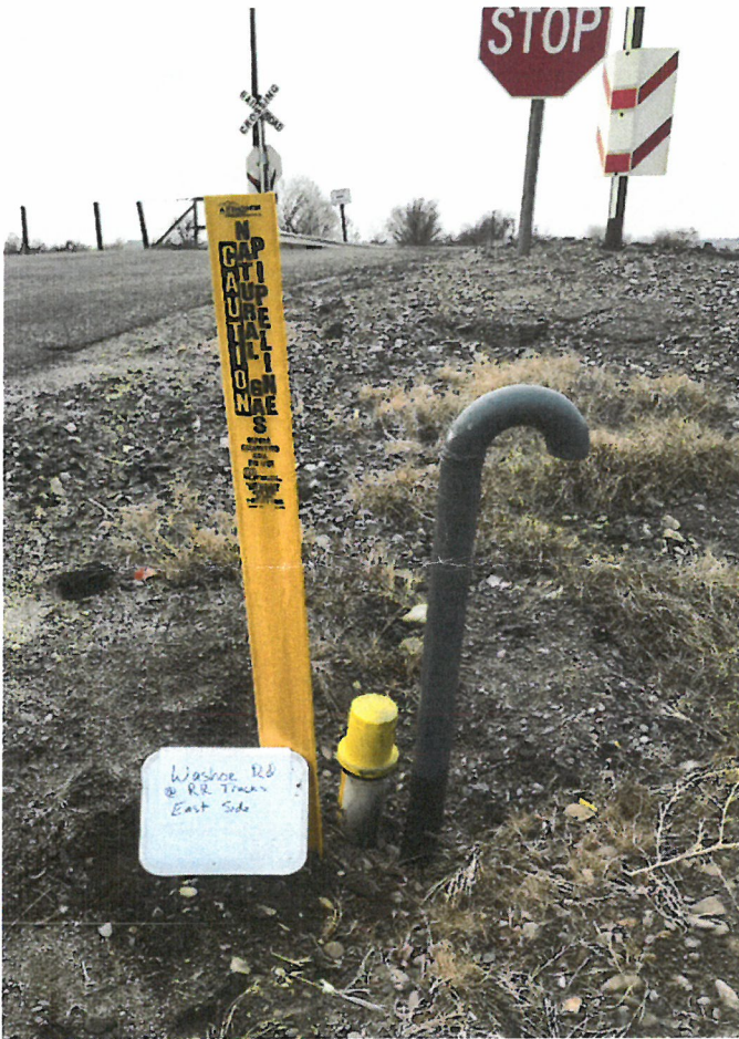
Figure 2: Vent Stack for Casing 26701306 (East Side)
