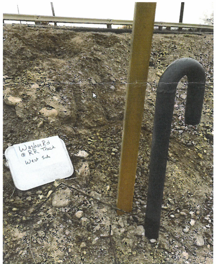
Figure 3: Vent Stack for Casing 26701306 (West Side)
